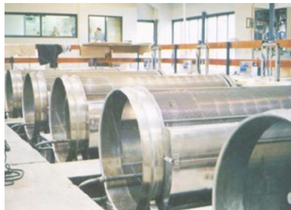
Figure 2: Micro-screens for floatables and small solid particles removal.
